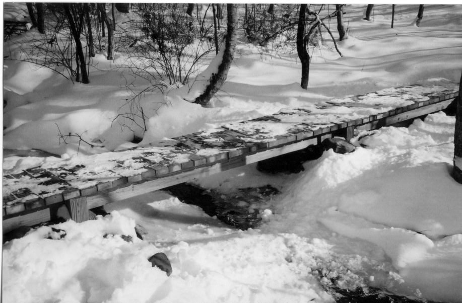
This new wetlands crossing bridge at the Byles Sanctuary in Mansfield was built by Eagle Scout candidate Nicholas Waleszczk under the guidance of retired E.O. Smith science teacher Bill O'Keefe.
